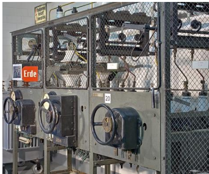
6-kV-switchgear in the exhibition
